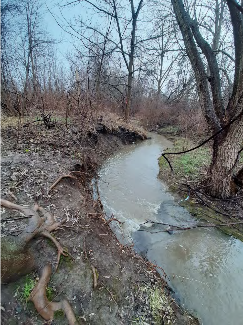
Figure 6: Photo of erosion on south bank of Shriners Creek.
