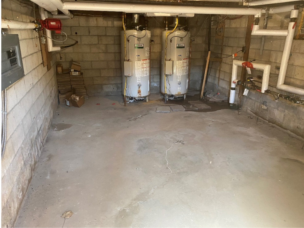
Photo 7: Basement Electrical Room (looking W).
