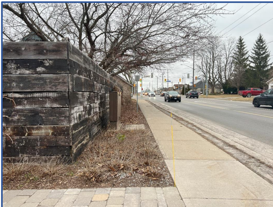
Photo 2 – View northward from driveway of 2495 Stanley Avenue. Stone shed located on 2358 Portage Avenue and encroaching into Stanley Avenue road allowance is visible (distant centre).
