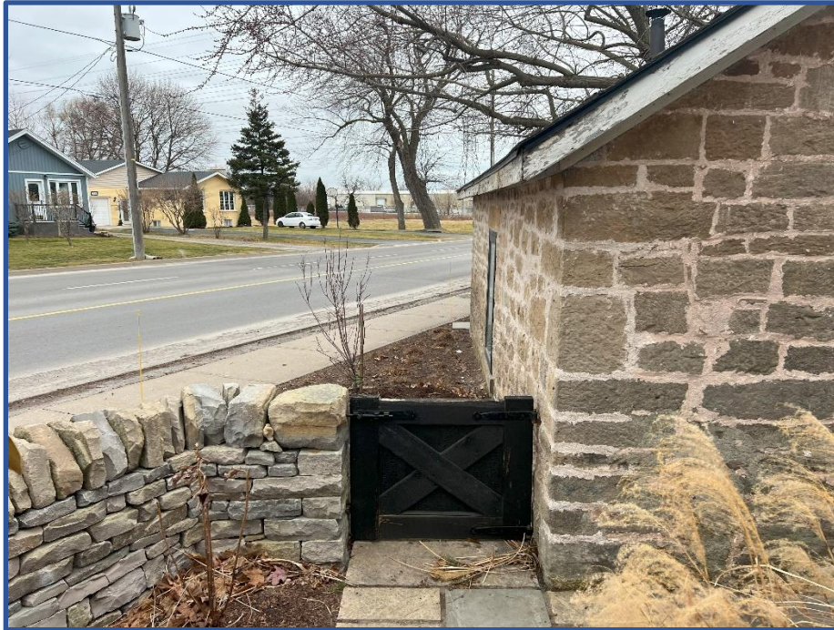
Photo 7 – View of stone shed from exterior side yard of 2358 Portage Road, looking southeast toward Stanley Avenue.
