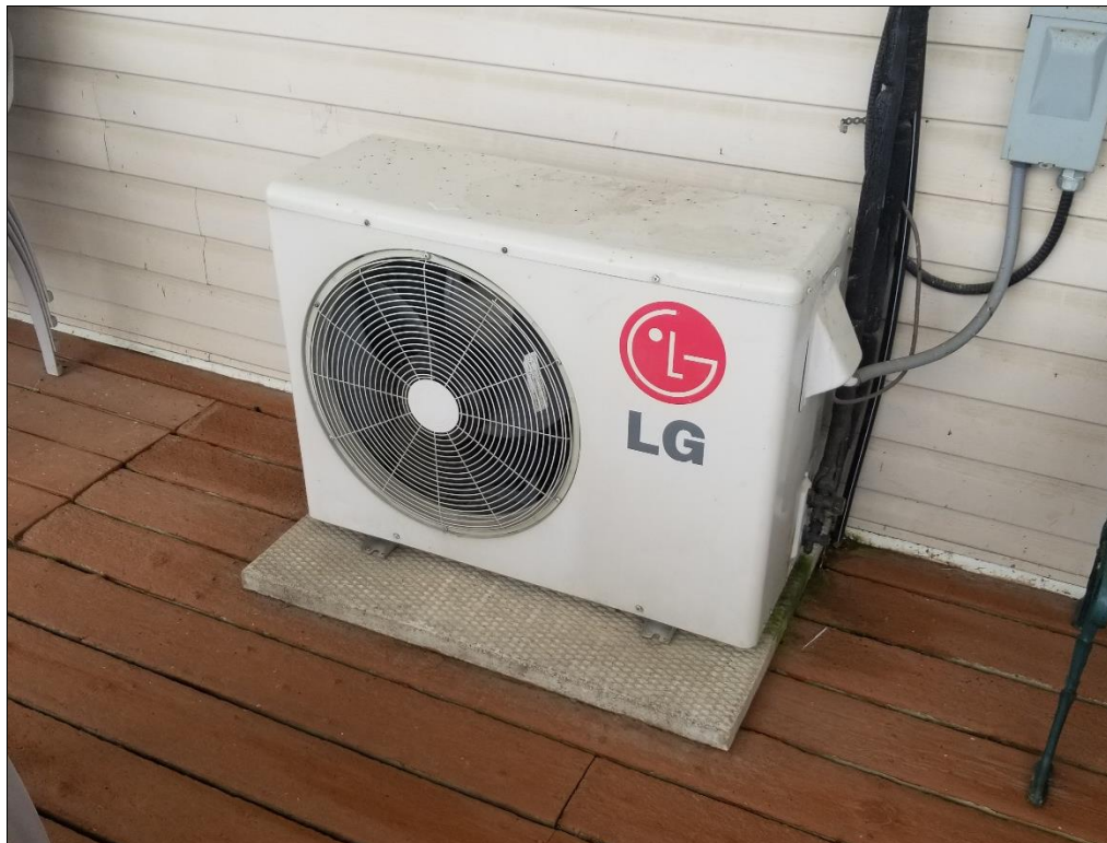
Photo 8: Electric heat pump Date: January 24, 2019 Direction: -
