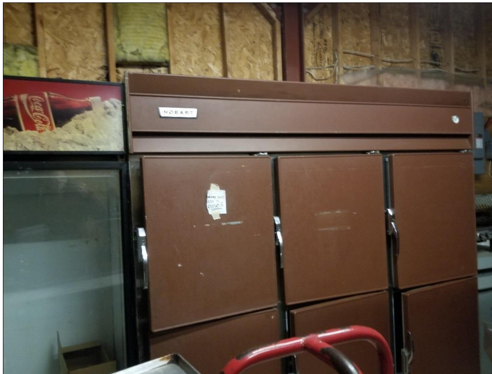
Photo 6: Old refrigeration units no longer in use
