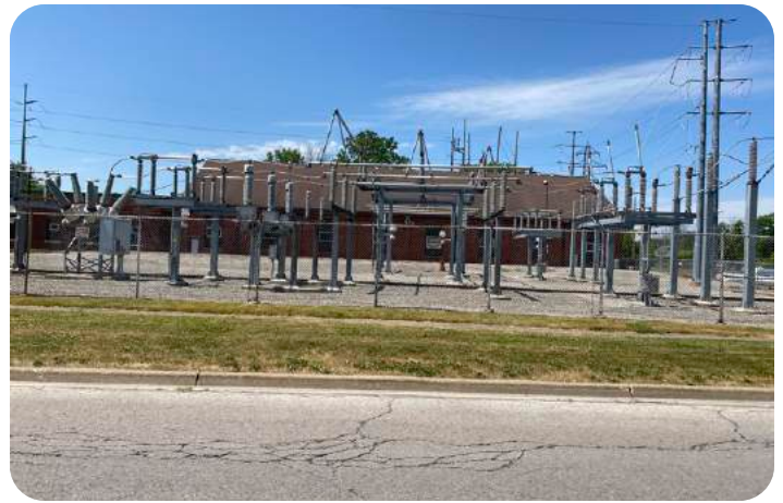
View of hydro transformer south of site
