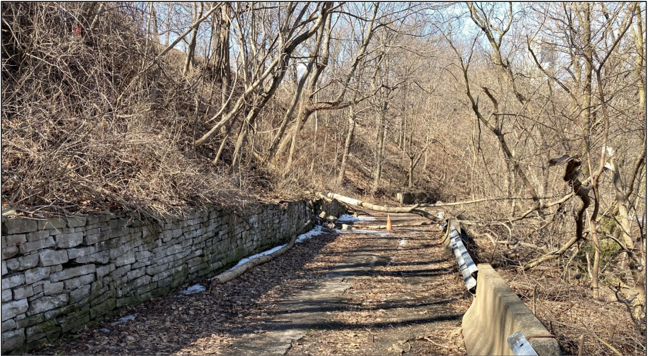
Photo 3: Facing downslope on the Fraser Hill road, currently closed to traffic and pedestrians. Note the steepness of the moraine slope, the stone retaining wall to the left, and the safety guardrail to the right.
