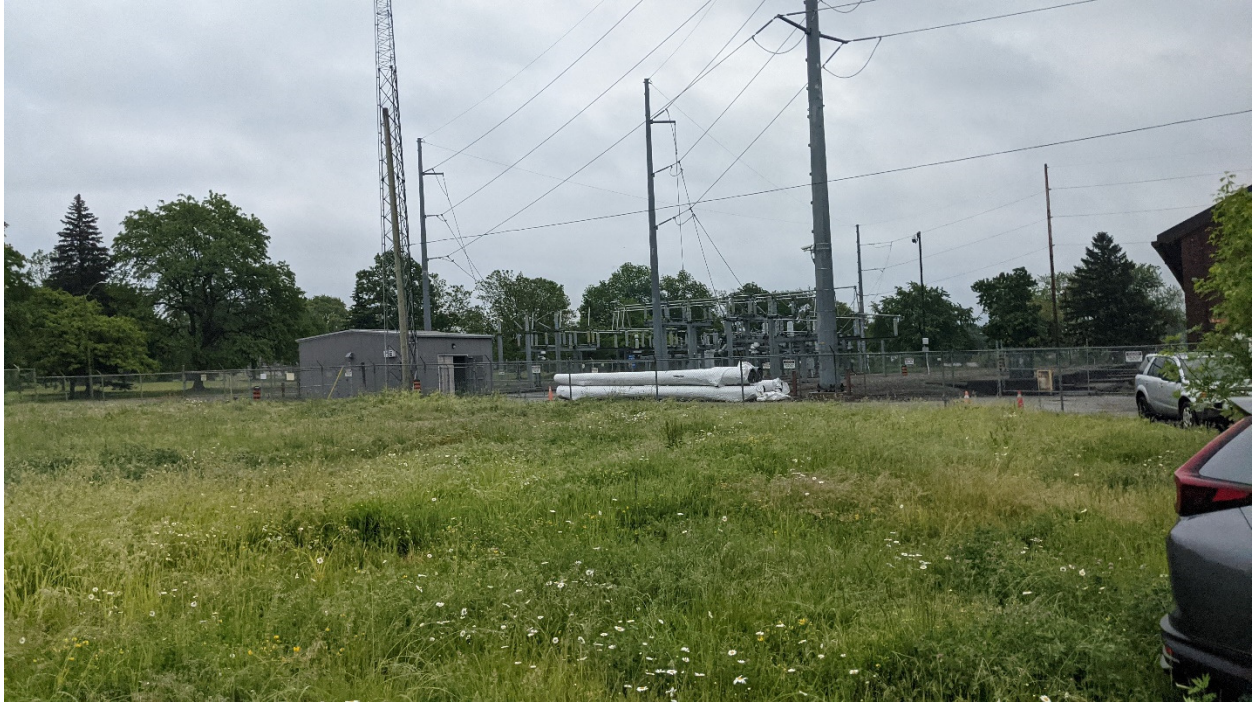
A view of the adjacent hydro transformers, from the south end of the Site, facing southeast.
