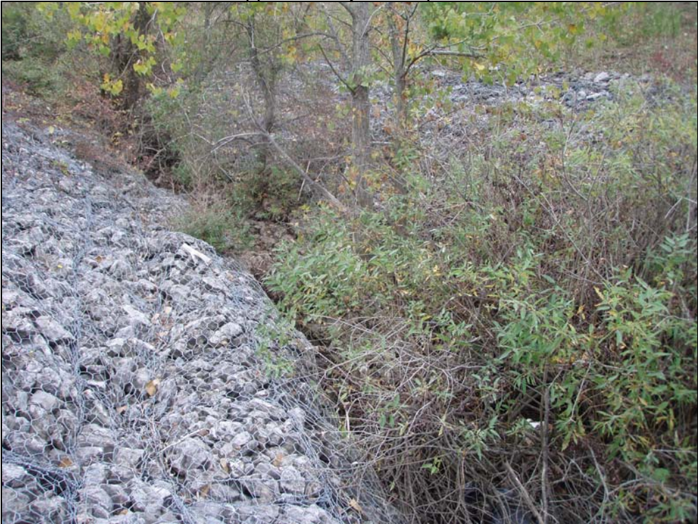
Photograph 10. October 6, 2015. Collapsed rock-filled gabions in sloped section of Watercourse 3, approximately 30 m upstream from mouth.
