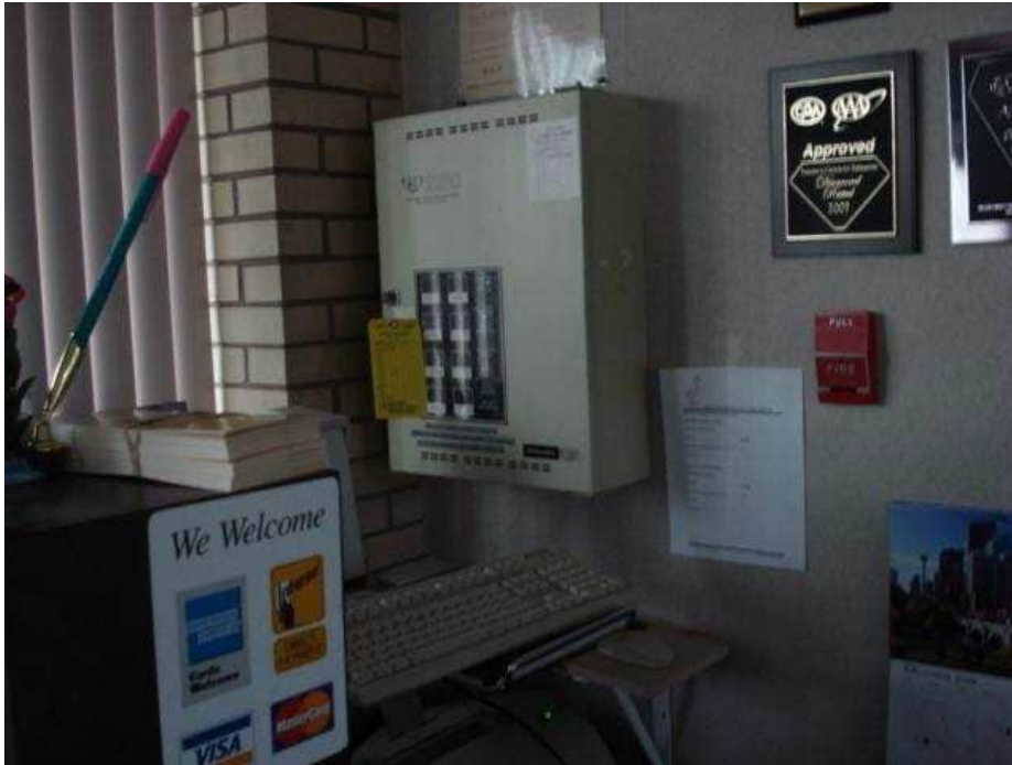
Annunciator Panel in Office
