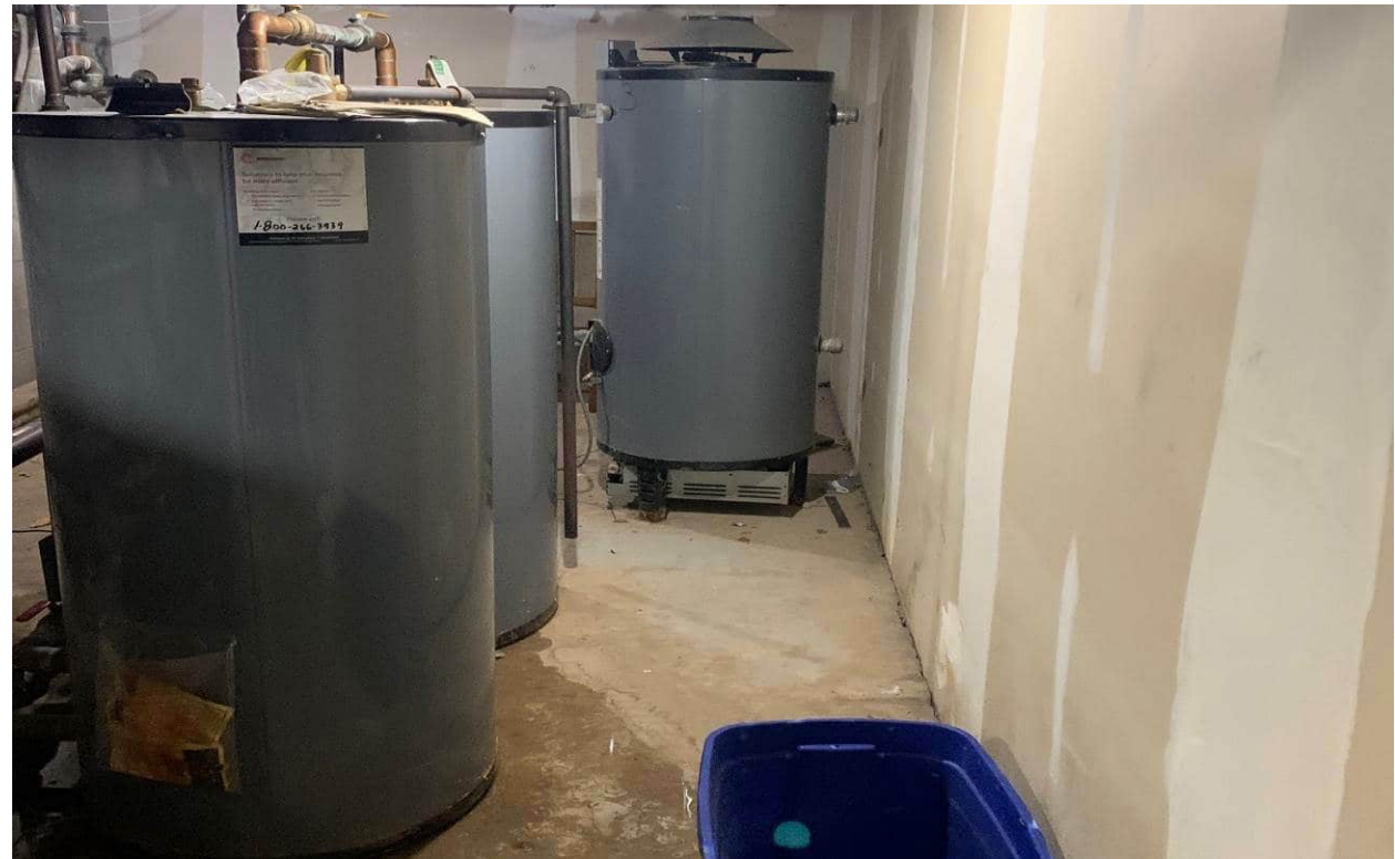
Photograph No.11 – Furnace room.
