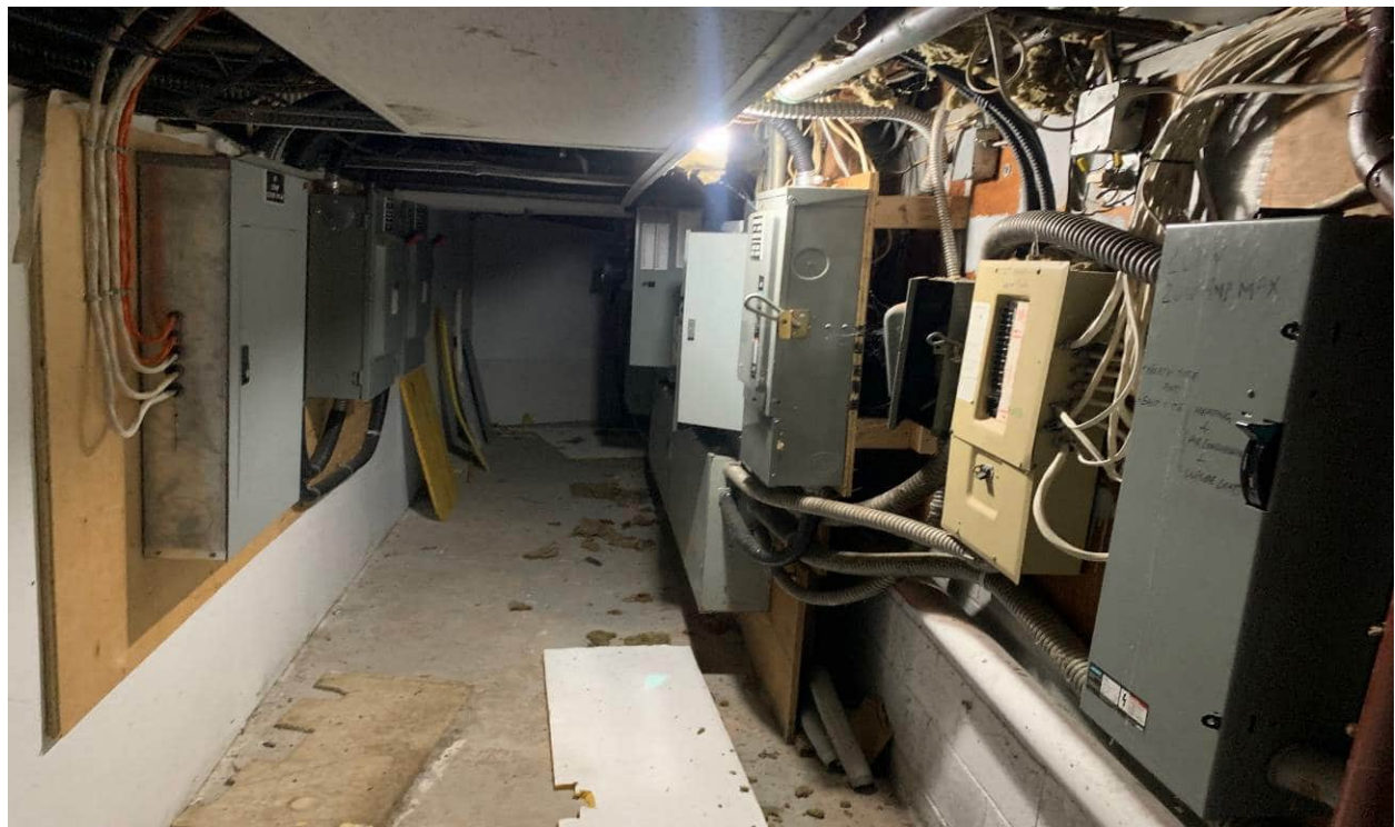
Photograph No.10 – Electrical room.
