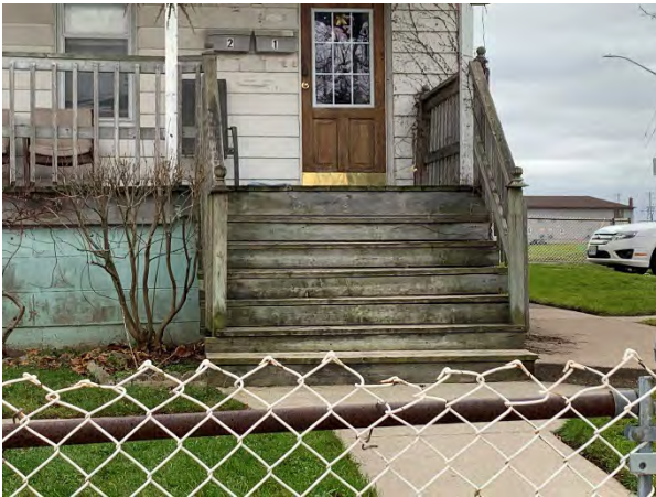
Plate 28 View of modern wooden stairs on northern elevation of the structure, facing south.
