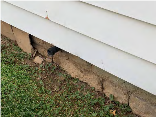
Plate 37 View shows where parking is failing along the south elevation of the structure revealing rusticated concrete below, facing northwest.
