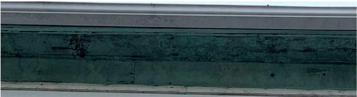
Plate 36 View of the eave along the south elevation. This image shows that the decorative pattern has been removed here. Faint marks are visible where the floral inlay was once present.
