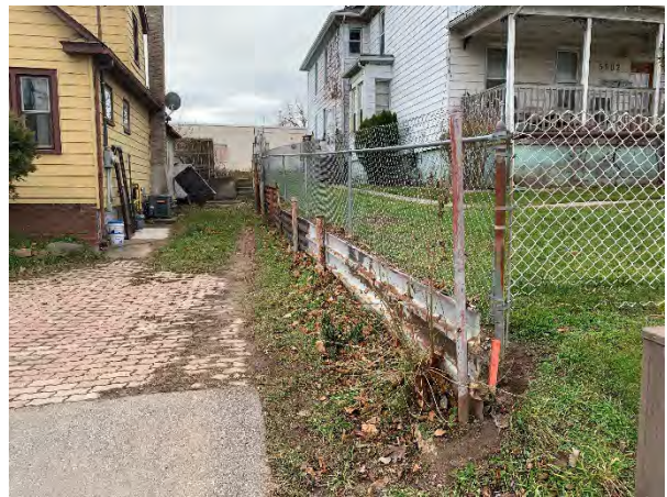
Plate 21: View showing raised grade of the Study Area supported by a retention wall on the east side of the residence, facing south.
