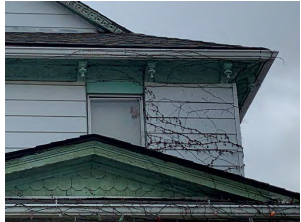
Plate 31 Detail on the second floor and roof of the northern elevation, facing south.
