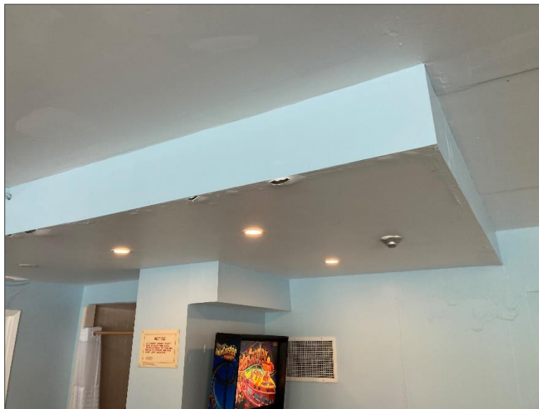
Photo 14 – Representative view of water damage within the pool room of the Site Building.
