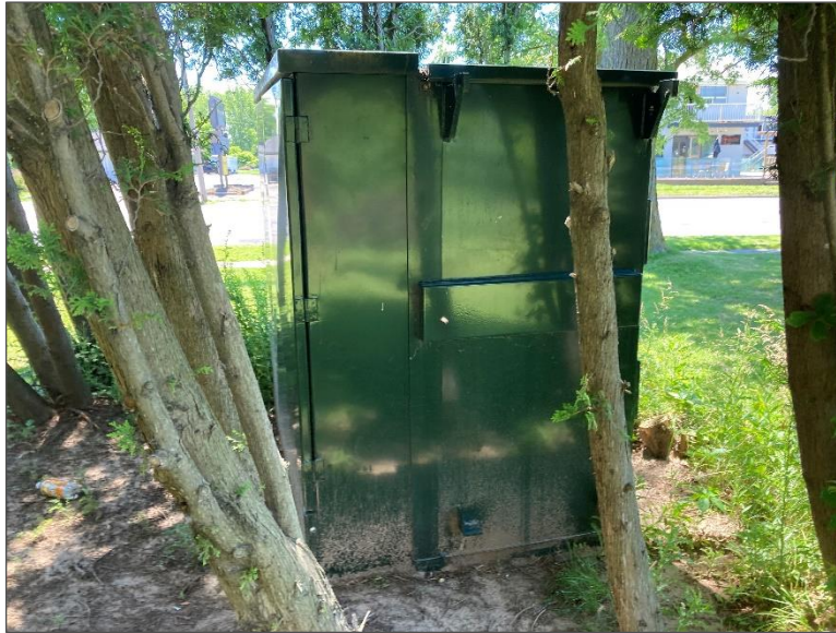
Photo 19 – View of pad-mounted transformer located on the southwest corner of the Site.
