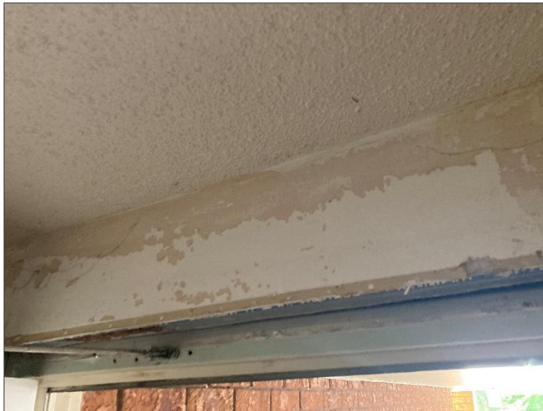
Photo 16 – Example of chipped and flaking paint within the Site Building.
