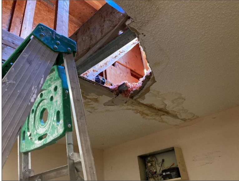
Photo 15 – View of water-stained building materials in the vicinity of the roof access.
