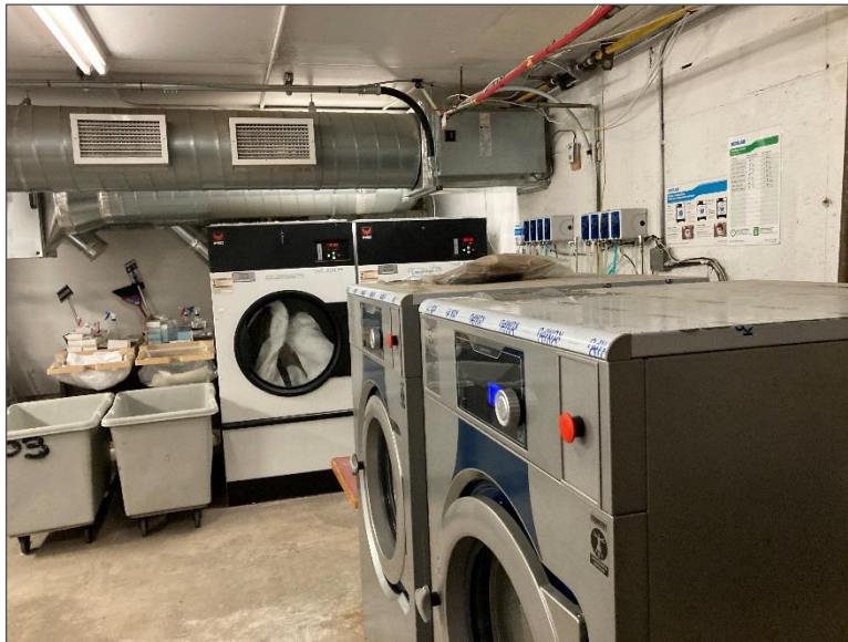
Photo 12 – View of the laundry room within the basement of the Site Building.
