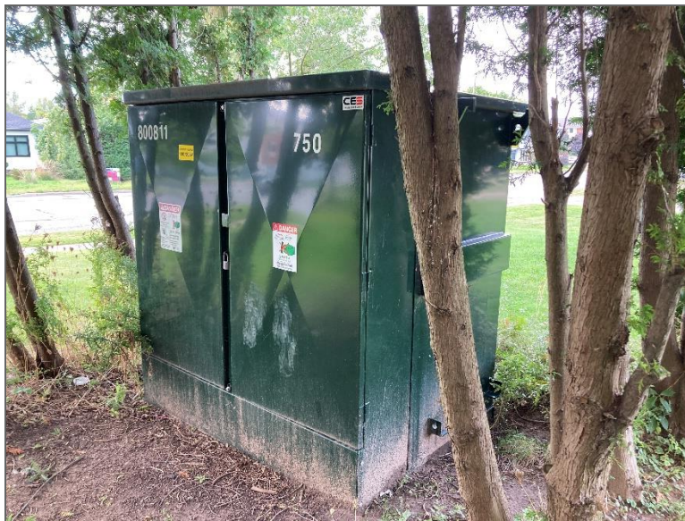
Photo 10 – View of pad-mounted transformer located on the southwest portion of the Phase One Property.
