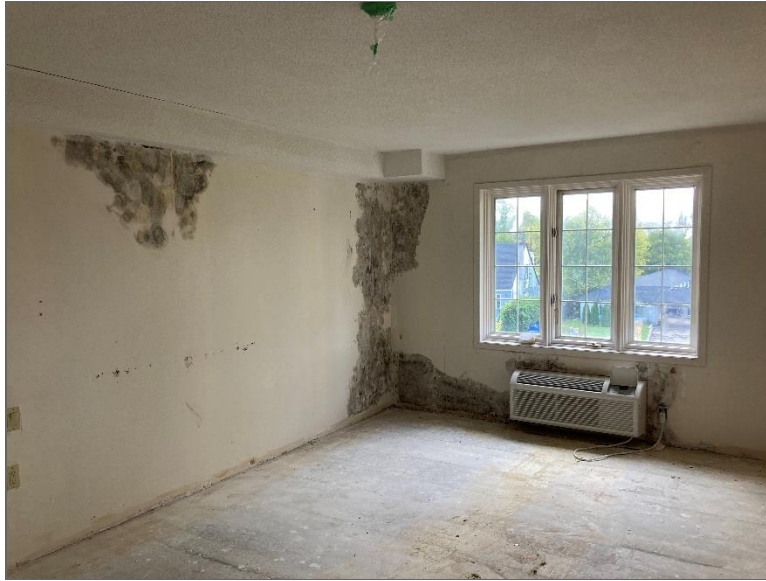
Photo 17 – View of water damage within a suite on the third floor of the Site Building. .
