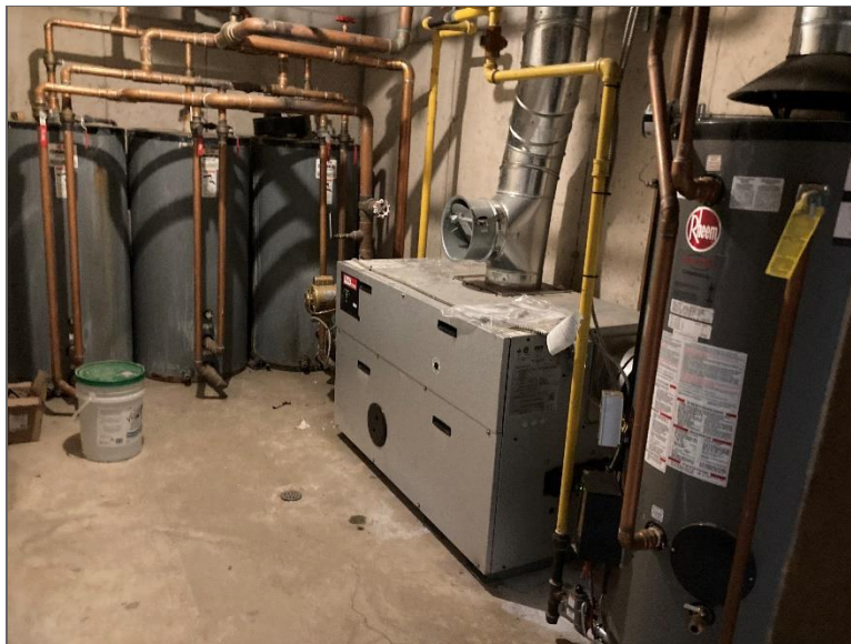
Photo 12 – View of boiler room in the basement of the Site Building.
