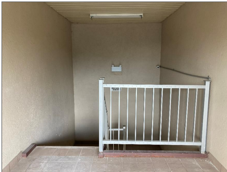
Photo 18 – View of exterior stairwell on the third floor of the Site Building.
