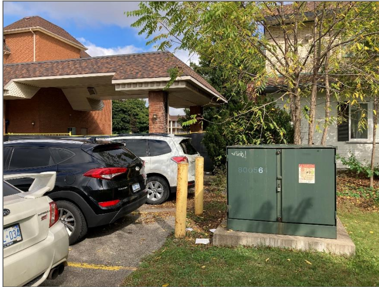
Photo 19 – View of pad-mounted transformer located on the property east adjacent to the Phase One Property.
