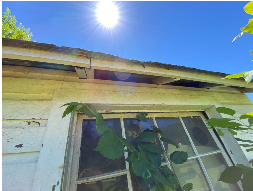
Photo 8: Gaps in the soffits of Outbuilding 1.
