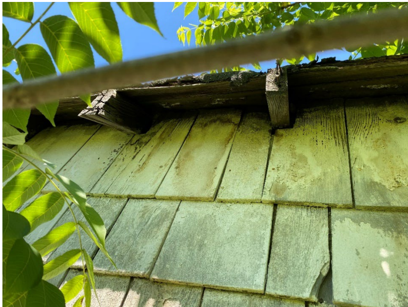
Photo 11: Gaps in the soffits of Outbuilding 2.
