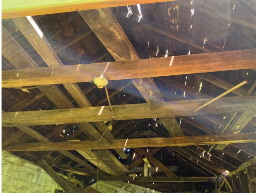
Photo 10: Gaps in the ceiling of Outbuilding 2.
