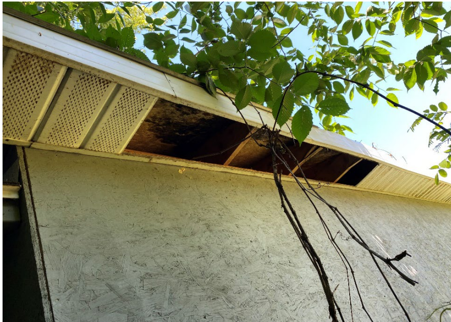
Photo 12: Gap in the soffit of Outbuilding 3.
