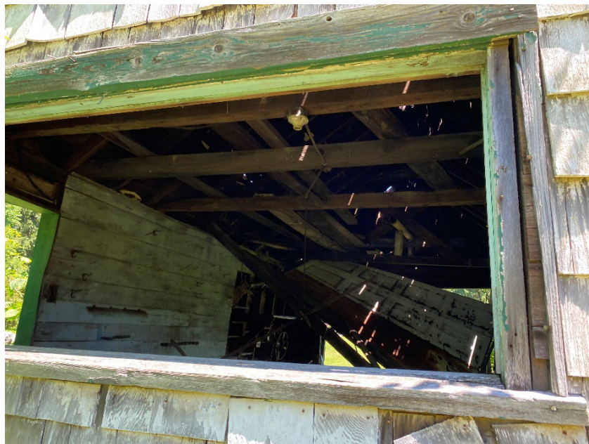
Photo 9: Open windows and doorways in Outbuilding 2.
