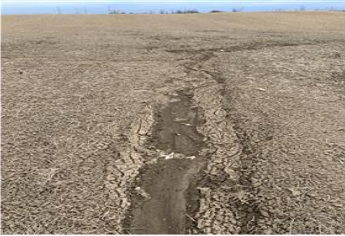
Photo 85: April 9, 2021 – Feature 21. Facing upstream (southwest)
