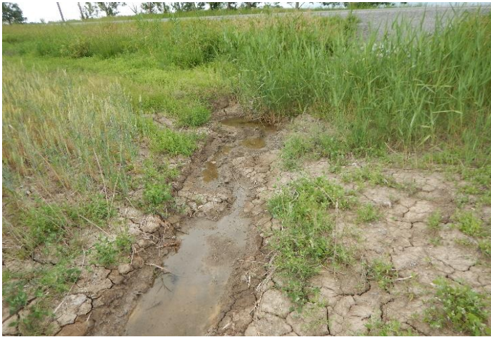
Photo 57: June 22, 2017 – Feature 10. Looking at east side of Thorold Townline Road facing upstream (west)
