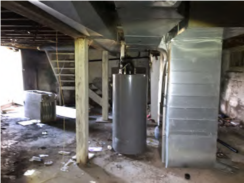
Hotwater tank and ductwork in basement of 5619 Murray Street, facing south
