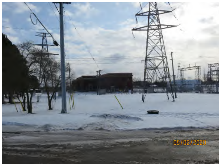
View of transformer station to the south, facing south
