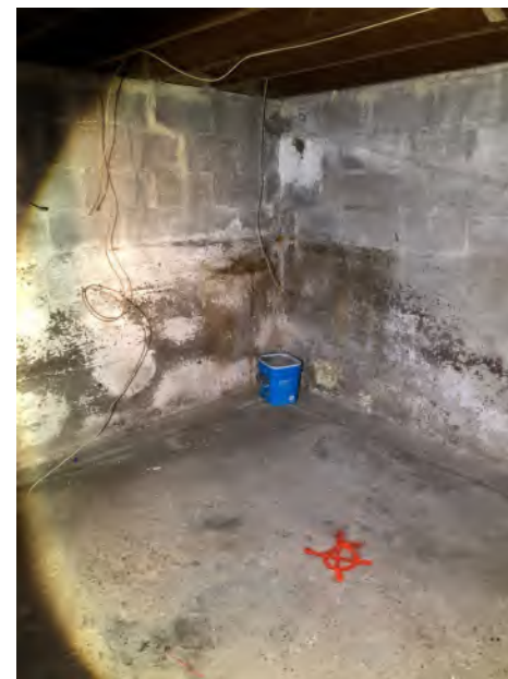
Former vent and fill pipes on the northeast corner of the basement at 5619 Murray Street
