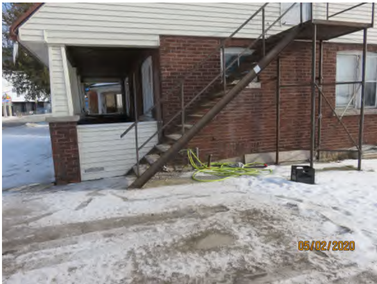
Vent and fill pipes on west elevation of 6285 Main Street, facing east
