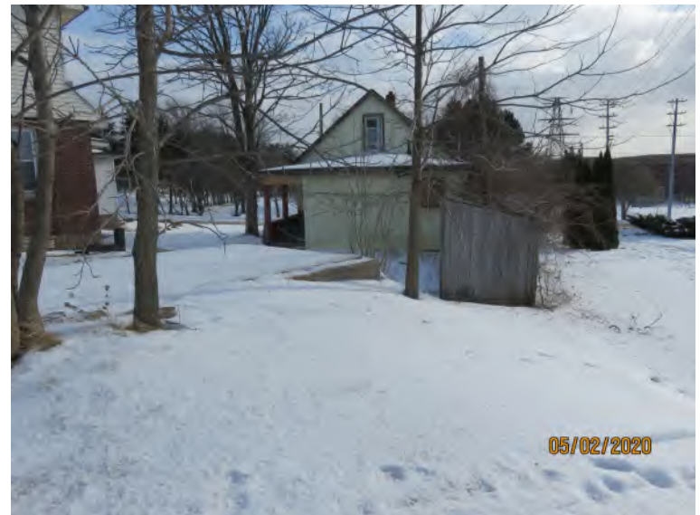
View of former auto shed concrete slab at northwest corner, facing south
