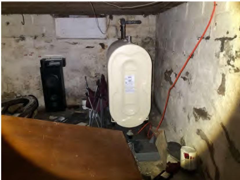
Aboveground fuel oil tank with vent and fill pipes on the northwest corner of the basement at 6285 Main Street
