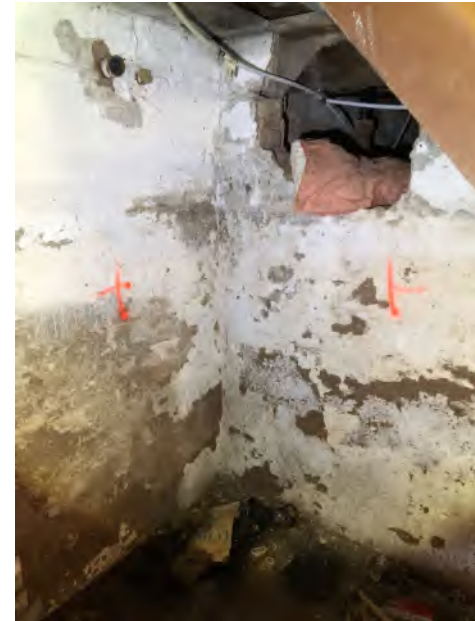
Former vent and fill pipes on the northwest corner of the basement at 5643 Murray Street
