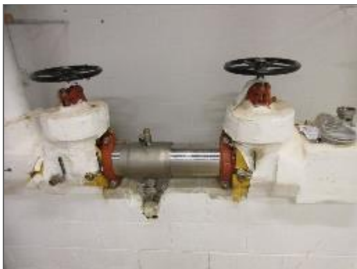
View of the backflow prevention device installed onto the main water line.
