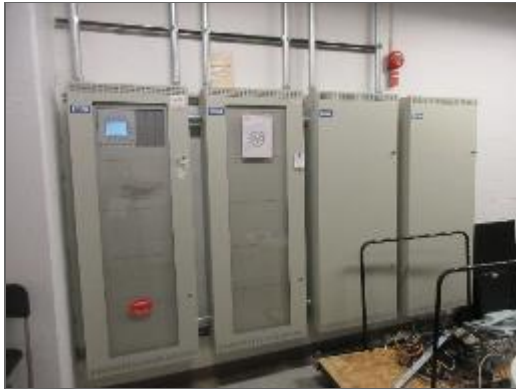
General view of the main fire alarm panel in the main service room.
