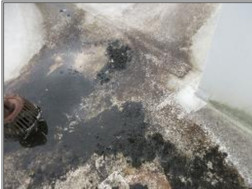
View of the organic debris accumulation atop the roof system.
