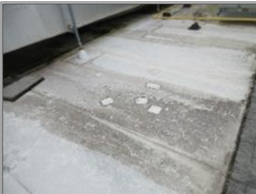
View of previous repairs/patches on the TPO membrane.
