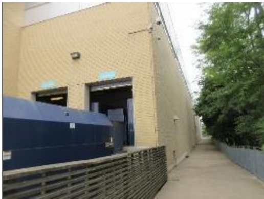
View of the brick veneer masonry on the south elevation of Site Building.
