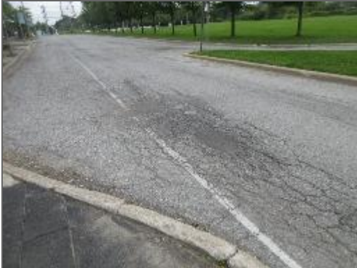
Typical view of alligator cracking at the north asphalt-paved parking area.
