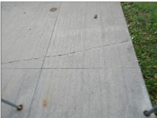
View of typical minor cracking noted in the concrete walkways.
