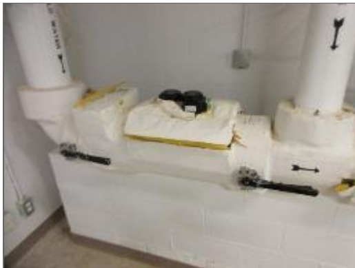
View of the main water line within the fire sprinkler room of the Site Building.
