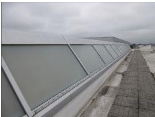
View of a typical skylight noted atop the north portion of the main roof system.
