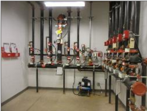
View of the fire sprinkler risers and shut off valves serving the Site Building.
