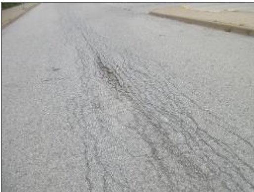
Typical view of alligator cracking at the west asphalt-paved parking area.
