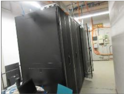
View of UPS system of the Site Building.
