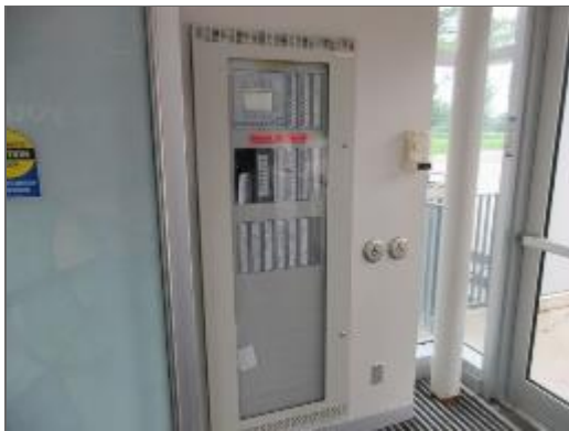
General view of the fire alarm annunciator panel at the main entrance.
