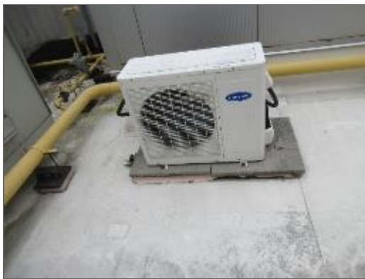
View of a typical air-cooled split condensing unit serving the Site Building.
