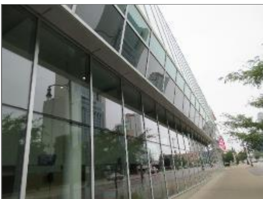
Typical view of the curtain wall systems noted on the east elevation of Site Building.
