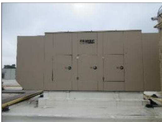
View of emergency generator of the Site Building.
