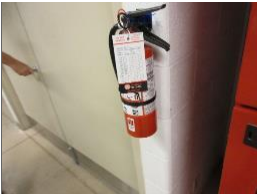
View of a typical fire extinguisher.
