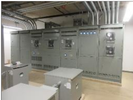
View of the main electrical switchgear unit serving the Site Building.
