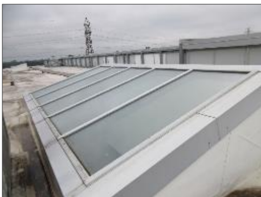
View of a typical skylight noted atop the north portion of the main roof system.
