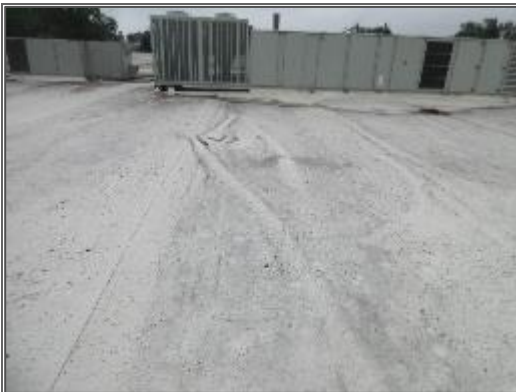
View of wrinkling in the TPO membrane.
