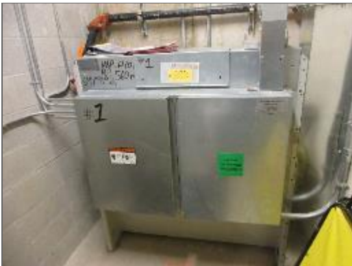
View of a typical hydraulic reservoir serving the elevators.
