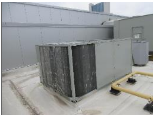
View of a typical rooftop HVAC unit serving the Site Building.
