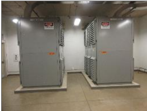
View of the concrete pad-mounted transformers serving the Site Building.
