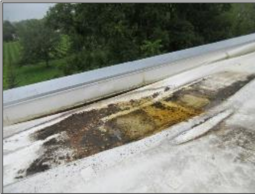
View of wrinkling and water ponding on the TPO membrane.
