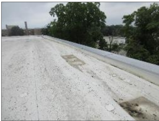
View of metal cap flashings at the roof parapet of the Site Building.
