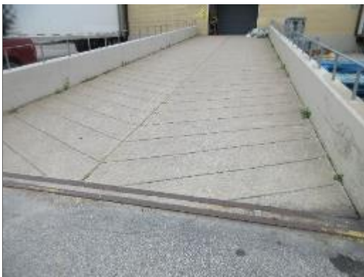
View of the concrete ramp and retaining walls adjacent to the west elevation of the building.
