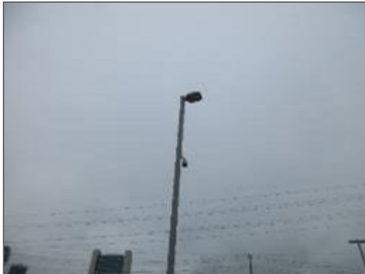
Typical view of exterior lighting at the Site.
