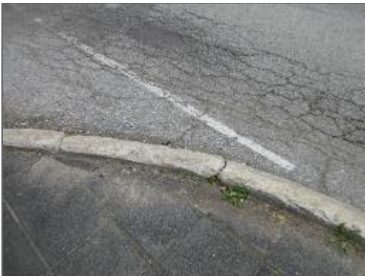
View of typical deterioration noted in the concrete curbs.
