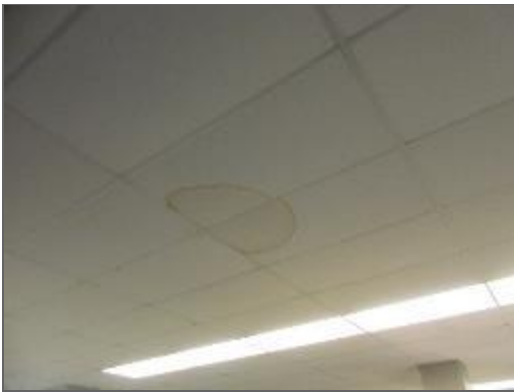
View of moisture-stained ceiling tiles in the office area of the Site Building.
