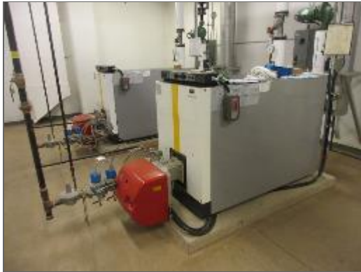
View of the heating boilers serving the Site Building.
