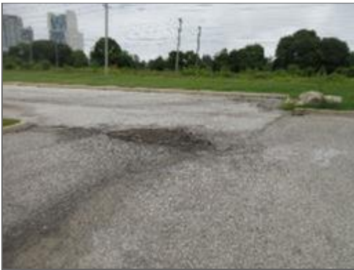
Typical view of deterioration and a pothole at the west asphalt-paved parking area.
