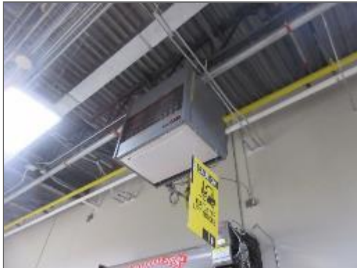
View of a typical suspended unit heater serving the Site Building.
