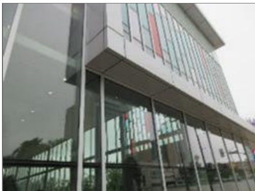
View of the metal wall panels noted on the north elevation of Site Building.
