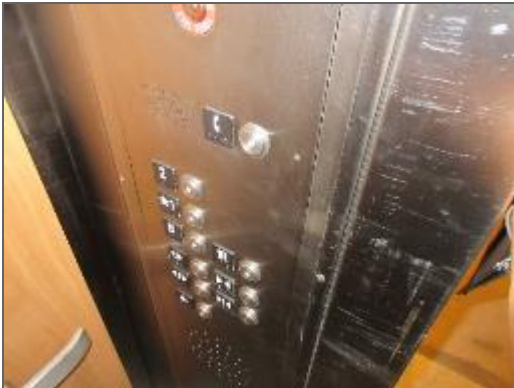
View of a typical elevator control panel.
