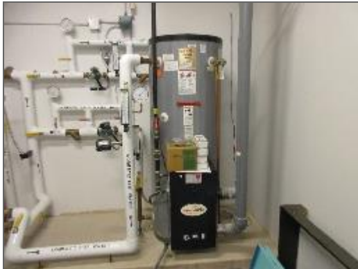
View of a typical DHW heater.
