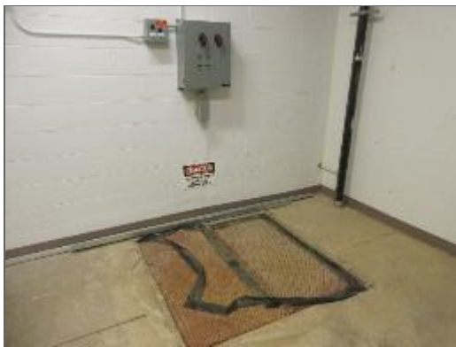
General view of the sump pump within the basement level of Site Building.
