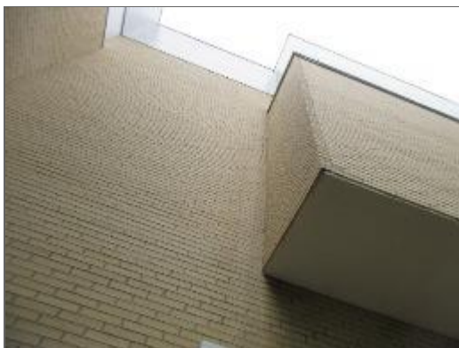
Close-up view of the brick veneer masonry on the south elevation of Site Building.
