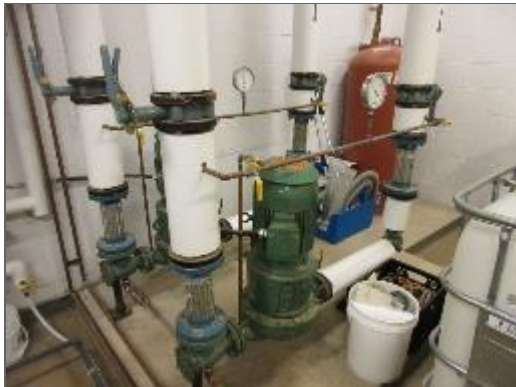
General view the circulation pumps serving the Site Building.
