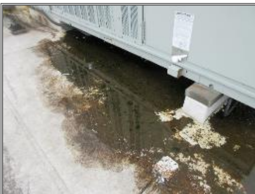
View of water ponding atop the roof system.
